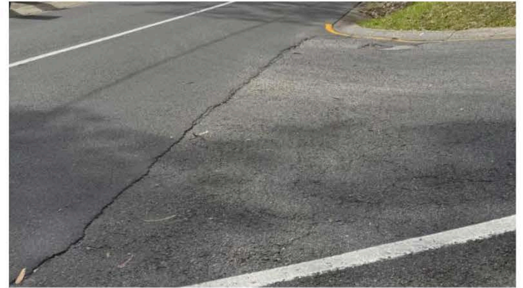
Pavement Condition on Ewers Avenue
