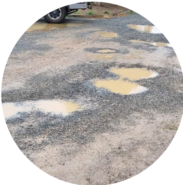
Uneven road surfaces
